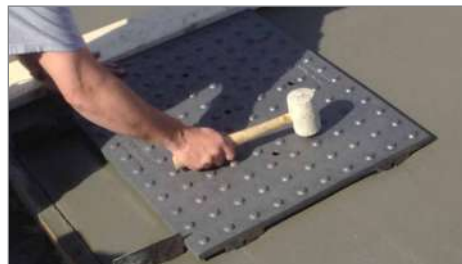
Tap plate in a grid pattern with a rubber mallet until concrete pushes through vents.
